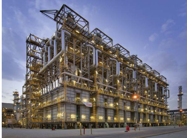
Photo from Linde Brochure: Seven ethane cracking furnaces by Linde Engineering North America for Saudi Ethylene and Polyethylene Company 4
